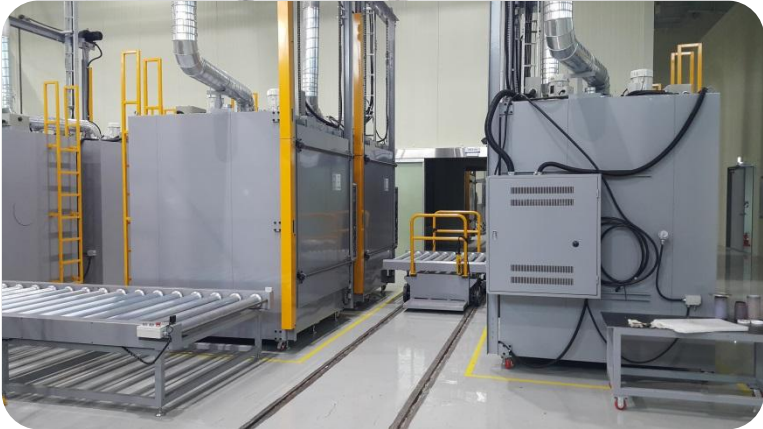
1st Curing Oven
