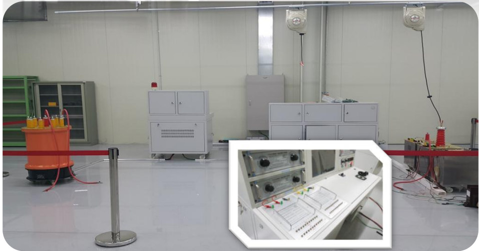
Accuracy & Inter Turn Over Voltage Test
