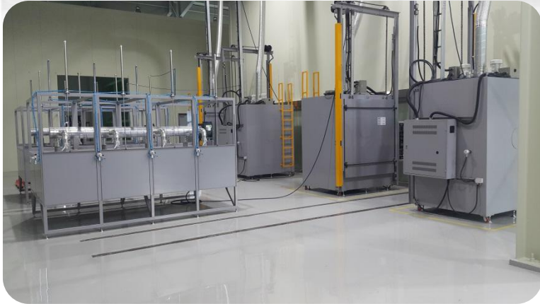
2nd Curing Oven
